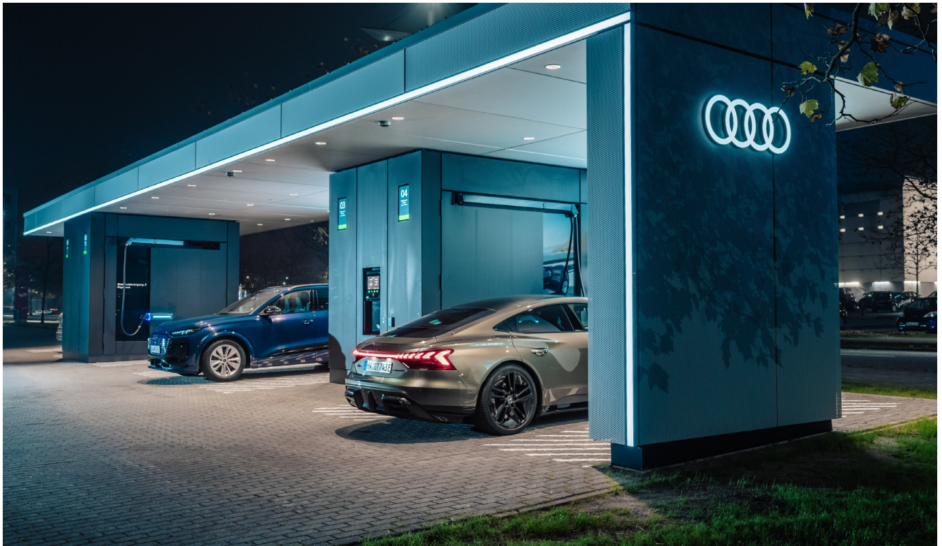
Audi charging hub in Bremen: Audi is setting a new milestone in the expansion of its urban charging infrastructure.
